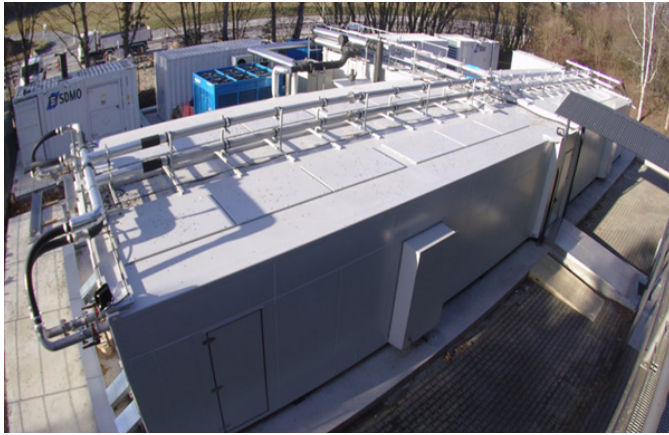
FIGURE 11. HPE Experience Center Geneva—4 x IT modules with a capacity of up to 84 IT racks in total, 2N redundant utility containers for power and chilled water
