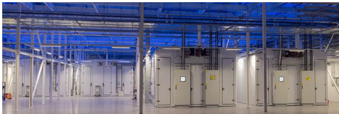
FIGURE 12. Warehouse data center farm—6 x HPE Performance Optimized Data Center DC44 with space of up to 20 units
